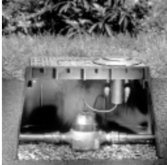
^ 50W-1 installed on pit meter
